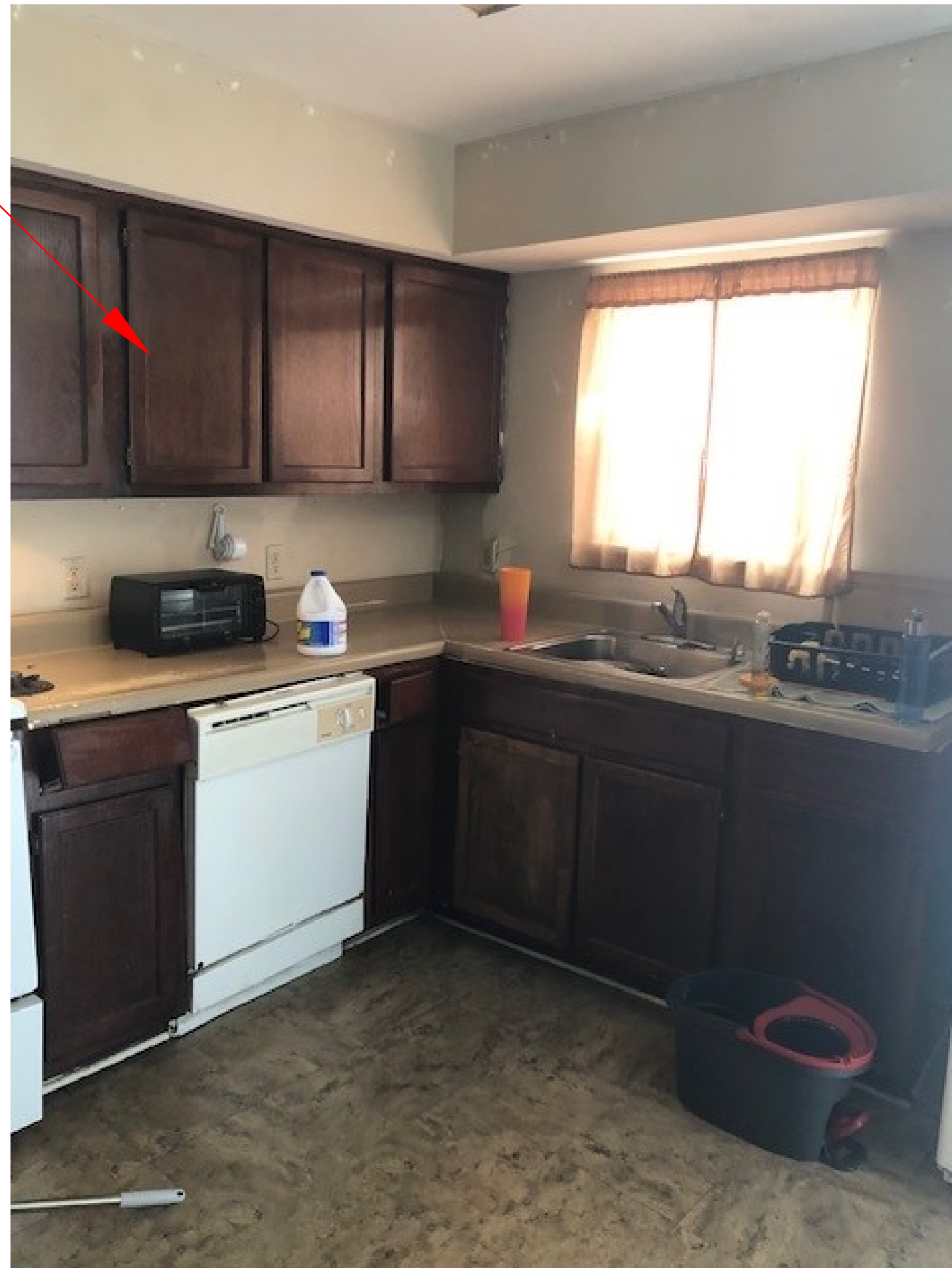
NORTHWEST CORNER DAMAGE
