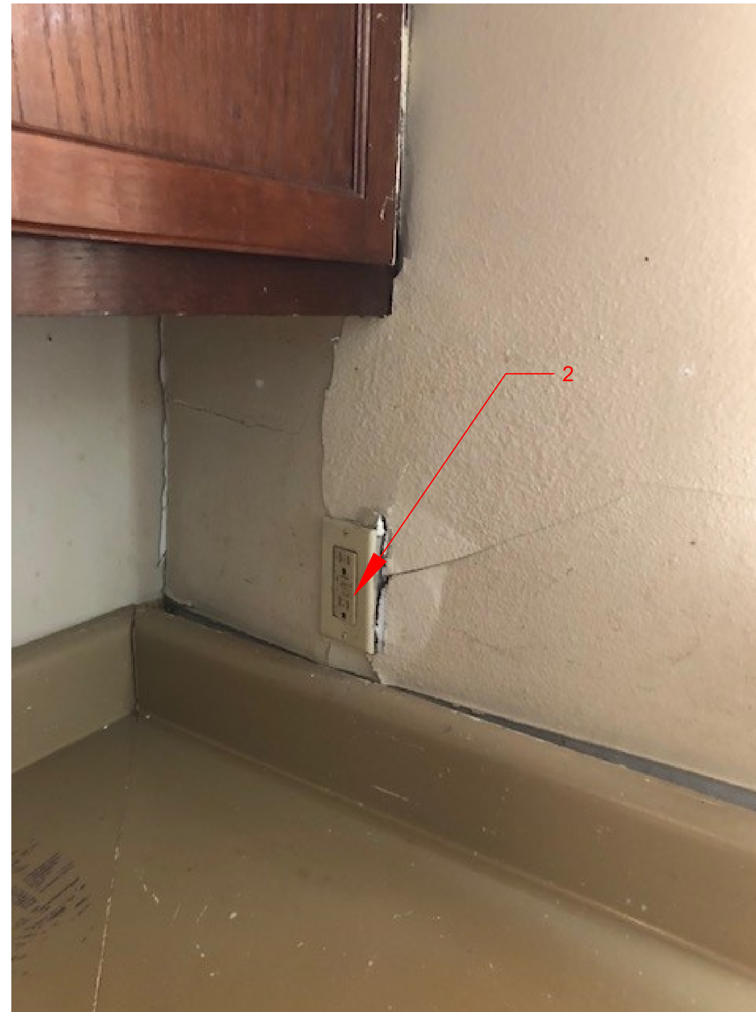
DETAIL OF NORTHWEST CORNER DAMAGE
