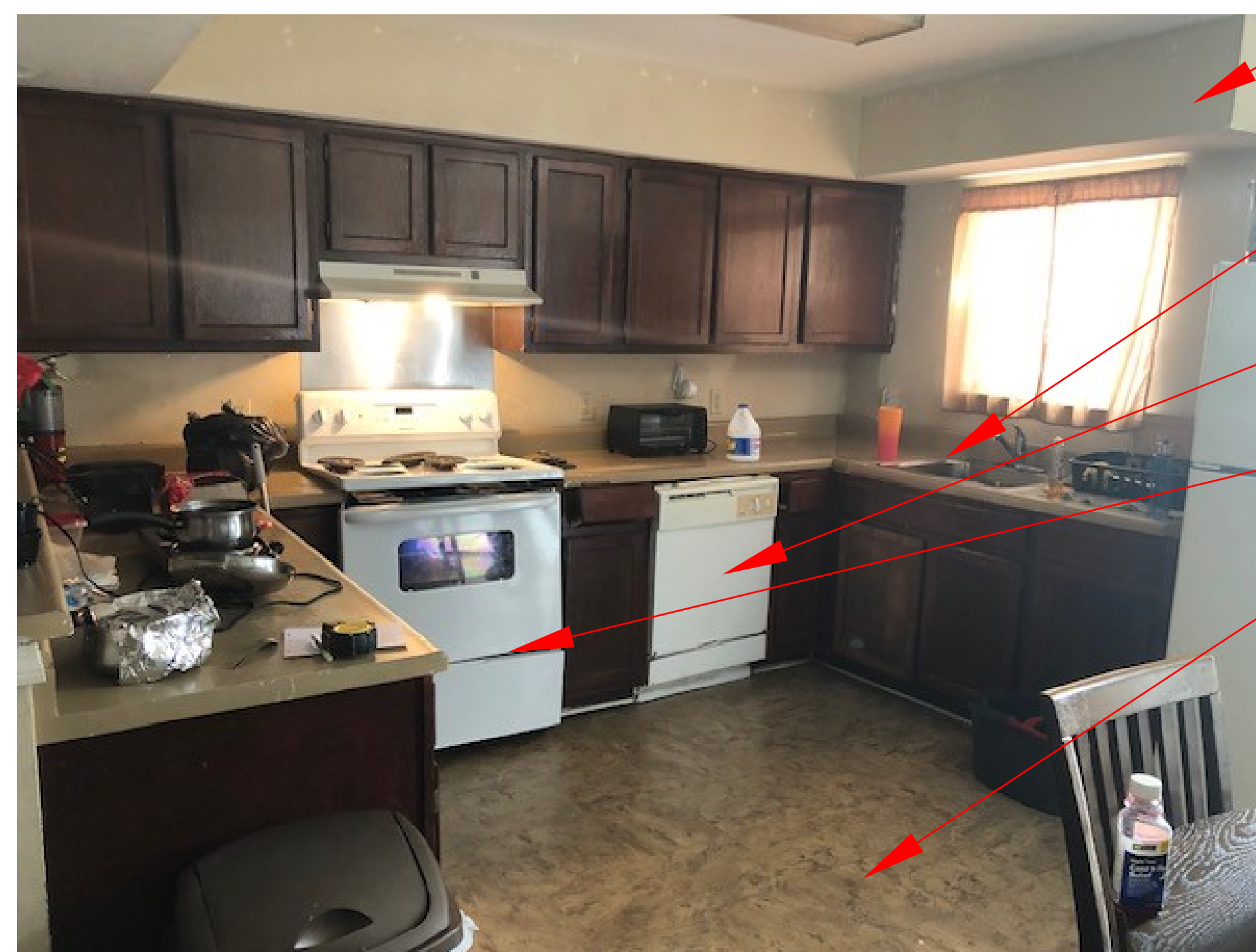
OVERALL VIEW OF NORTHWEST CORNER DAMAGE
