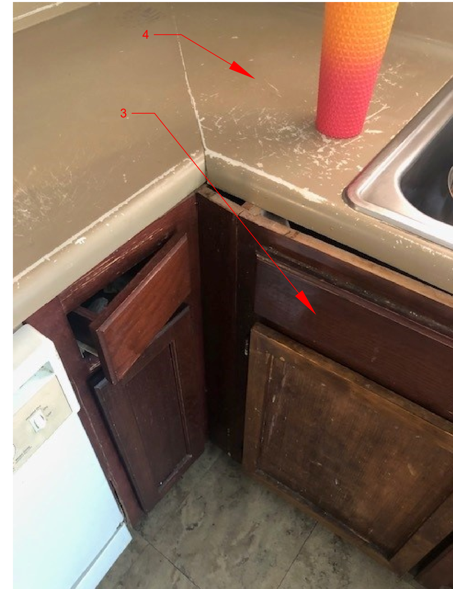
DETAIL OF NORTHWEST CORNER DAMAGE
